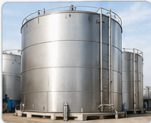
Storage Tanks & Utility Tanks
